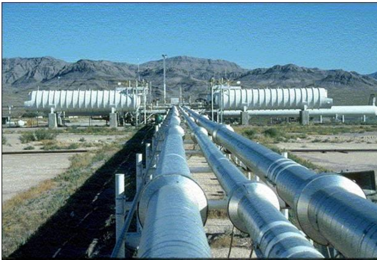
Figure 1 - Part of the tank farm used in the Kit Fox experiments, allowed for storage of large volumes of the surrogate dense gas released during the experiments – in earlier experiments up to 66m 3 of LNG was releases in about 2 minutes from these tanks and through these lines.
